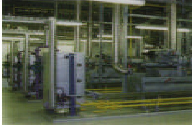
Machine room refrigerating plant
